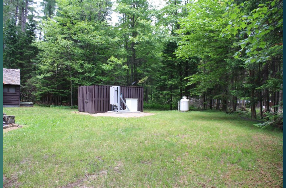
Generator & Lift Station – Day Use Area
