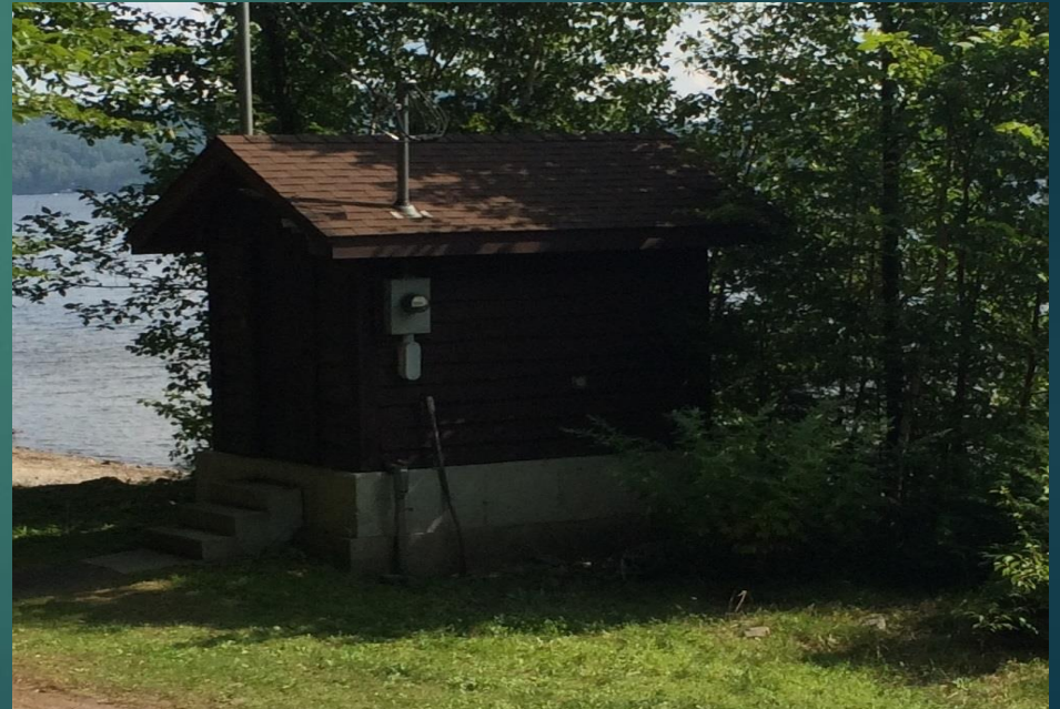
Water Pump House (16)
