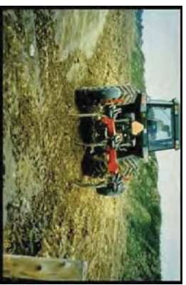
Fig. 9. This medium tractor is pulling a 3-shank deep ripper. The severely compacted construction access corridor is narrow, and the 120 hp tractor is more maneuverable for Phase 1 deep ripping (subsoil fracturing), here.
