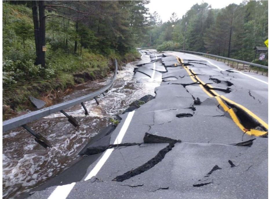
State Route 28N was closed in the Town of Long Lake after the heavy rains washed away roadway. Photo courtesy of Town of Long Lake
