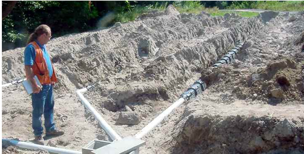
Larry Phillips conducts a compliance field visit for a subdivision violation. The owner was required to install a septic system designed to adequately work given the soil characteristics.
