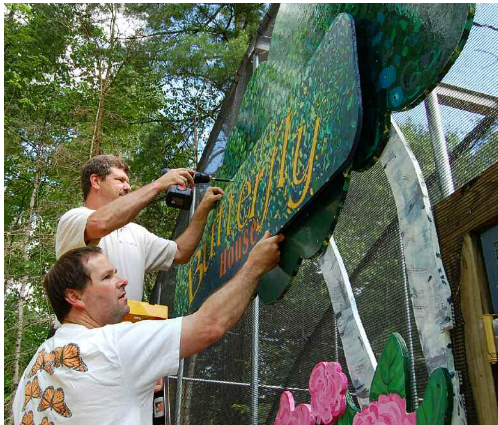
Environmental Educator Milt Adams holds the bottom of a sign as Maintenance Supervisor George Hare secures it to the front of the Native Species Butterfly House at the Paul Smiths VIC. Staff added a vestibule to the Butterfly House in 2007 to prevent butterflies and moths from escaping.
