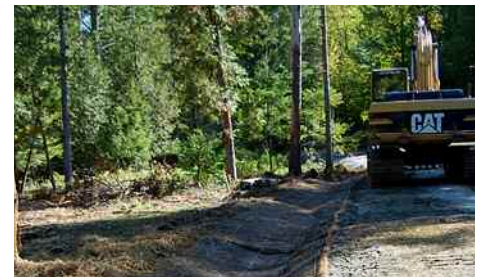
Porous matting is used on steep cell tower access roads to control stormwater runoff and to avoid soil erosion.
