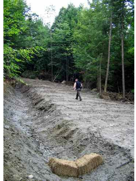
Enforcement Officer Joseph Thouin inspects a project site which involved an illegal stream crossing and wetland fill.
