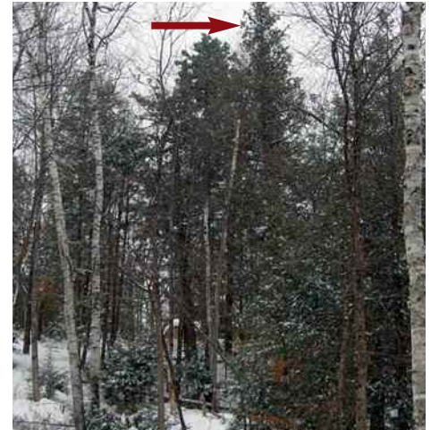
The arrow above shows a Verizon simulated white pine tree cell tower that provides coverage along the Adirondack Northway in the Town of Schroon.
