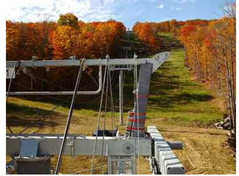
Here is some of the work on the new chairlift installation, as seen in the fall of 2008, which was part of the Burnt Ridge expansion at the Gore Mountain Ski Center in the Town of Johnsbury, Warren County.
