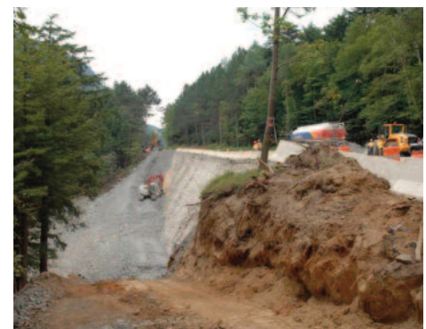
Emergency Authorization project to stabilize retaining wall in the Town of Keene, Essex County.
